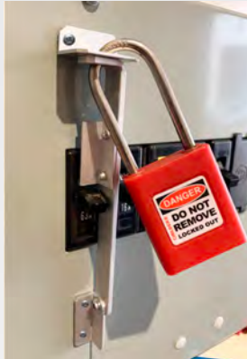
SALD-B-1 on Circuit Breaker
